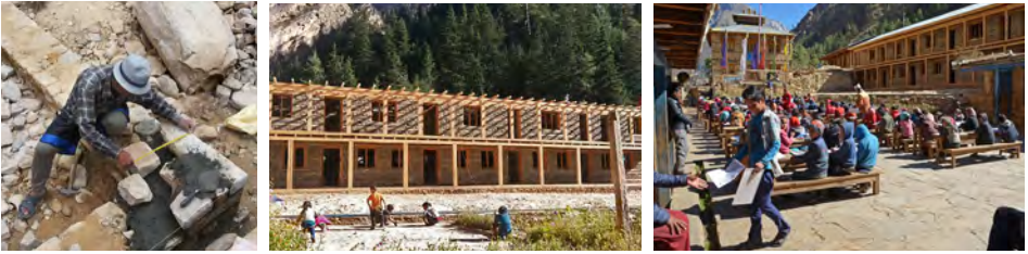
Reconstruction right wing: Reinforced corners with worked stones, building shell with wooden supports, exams in front of the new building © S. Lama, M. Kind
